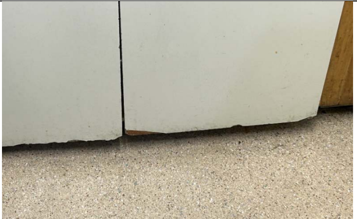
Chipped/worn out kitchen cabinetry
