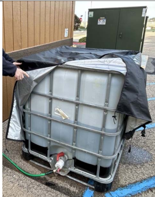
Non-potable water supply
