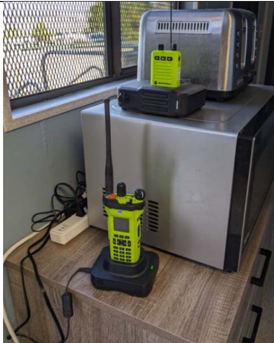
Alert system in modular trailer
