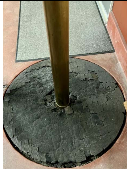
Poor condition of fire pole landing pad
